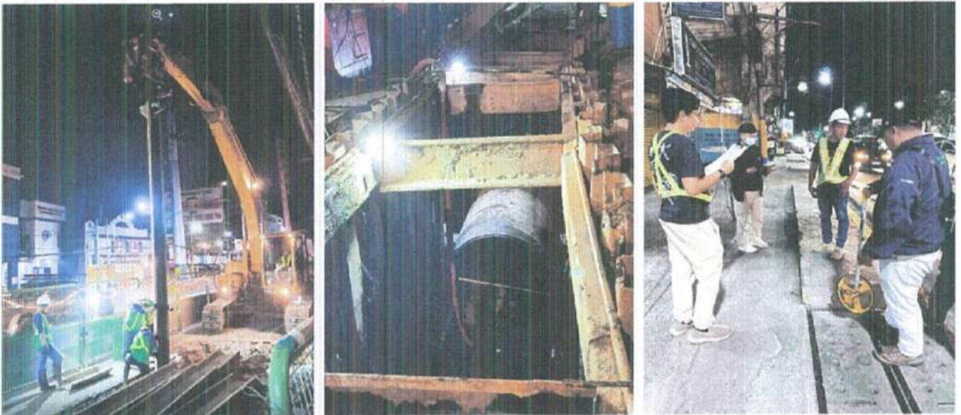
6 March 2026: Relocation of Maynilad Facilities for P2 & P3 at Aguinaldo Highway, Bacoor Cavite attended by LRТА-PMO, DOTr-PIU, and MAYNILAD
