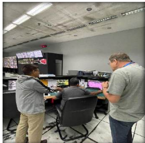
OCC Workstation for SCADA
