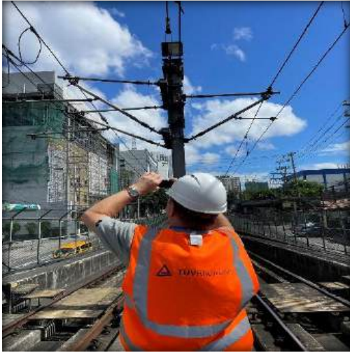
Overhead Catenary System
