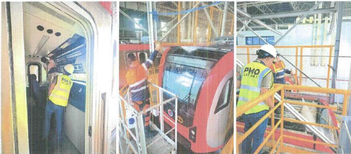
23 January 2026: Watertightness Test of Trainsets TS06 and TS10 represented by LRTA-PMO, DOTr-PIU, LRMC, CMX and MC-CAF
