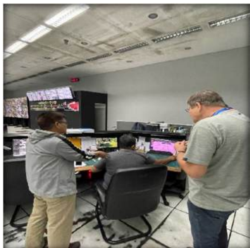
OCC Workstation for SCADA
