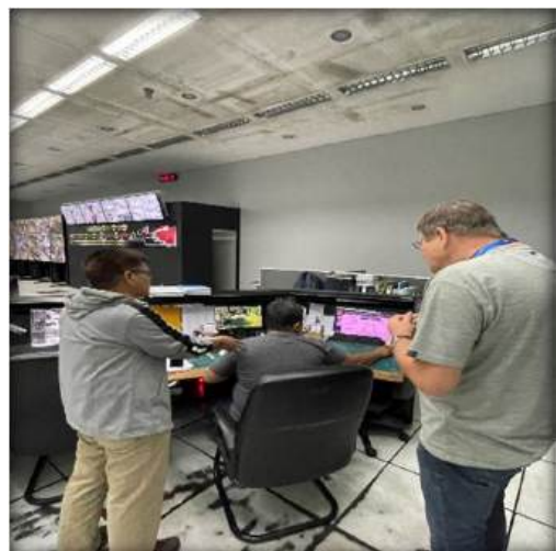
OCC Workstation for SCADA
