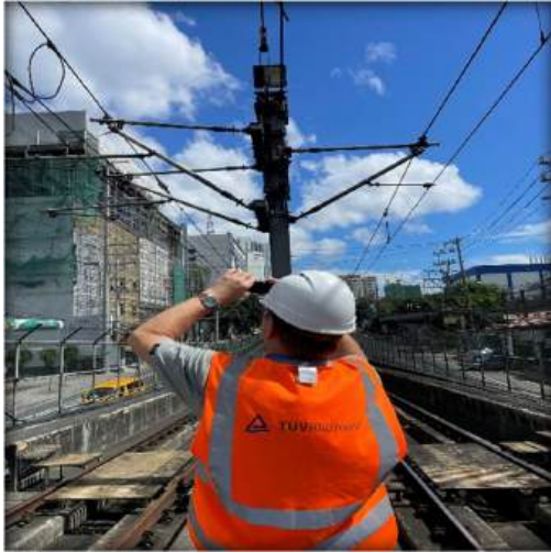
Overhead Catenary System
