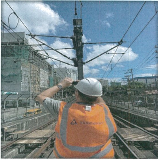
Overhead Catenary System
