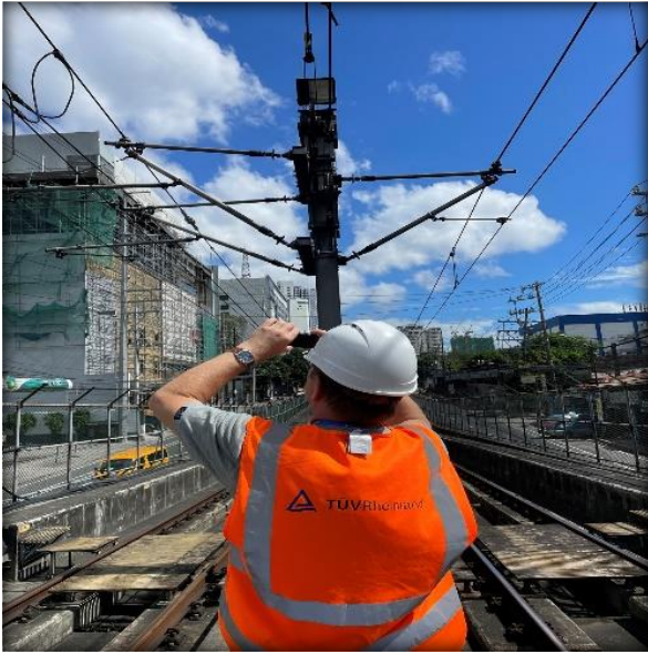
Overhead Catenary System
