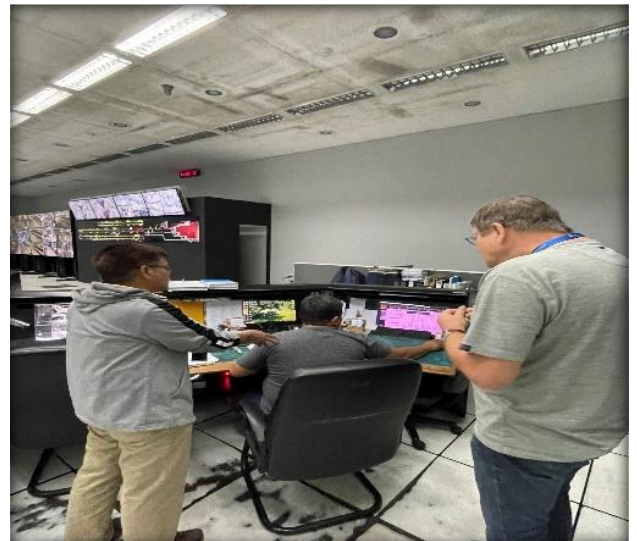
OCC Workstation for SCADA
