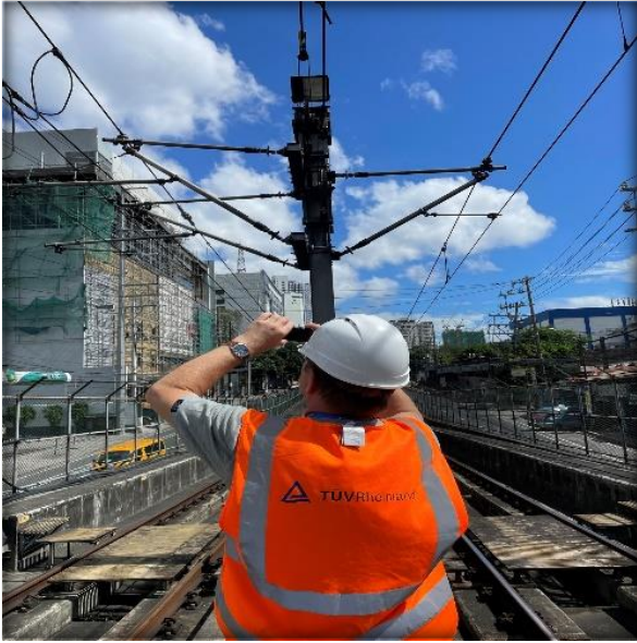
Overhead Catenary System
