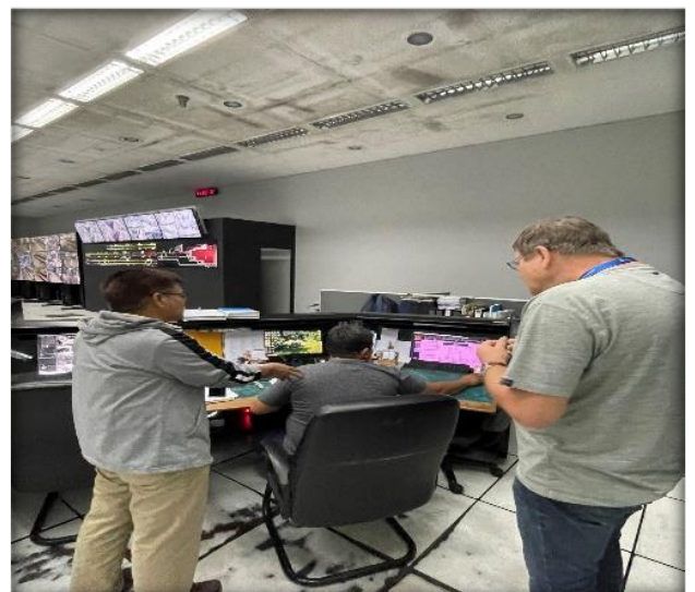
OCC Workstation for SCADA
