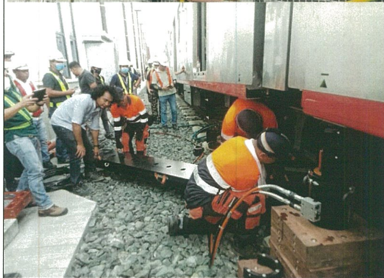
Expansion of the Existing Depot at Baclaran and Construction of New Satellite Depot at Zapote
