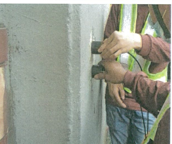
CRACK DETECTION ON PIER USING ULTRASONIC PULSE VELOCITY TEST
